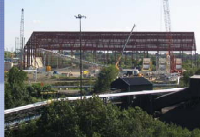
Schiller Station, NH (50 MW)
